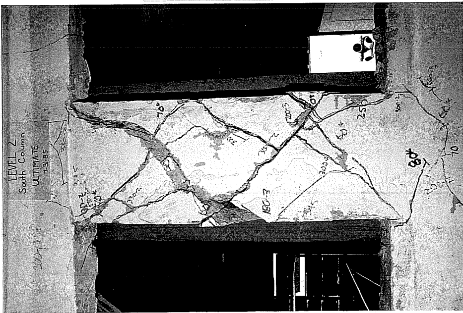
b) Shear failure of composite column
