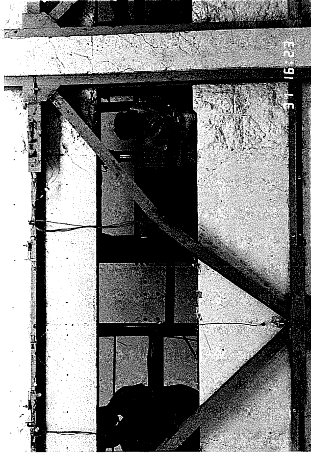
a) Buckling of brace
